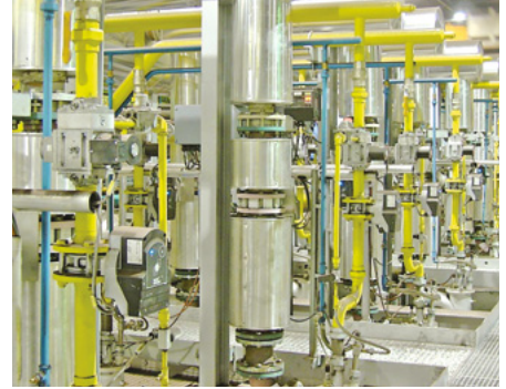
Walking beam furnace with overhead firing
